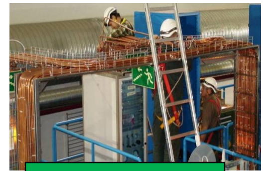
Muon Barrel piping
